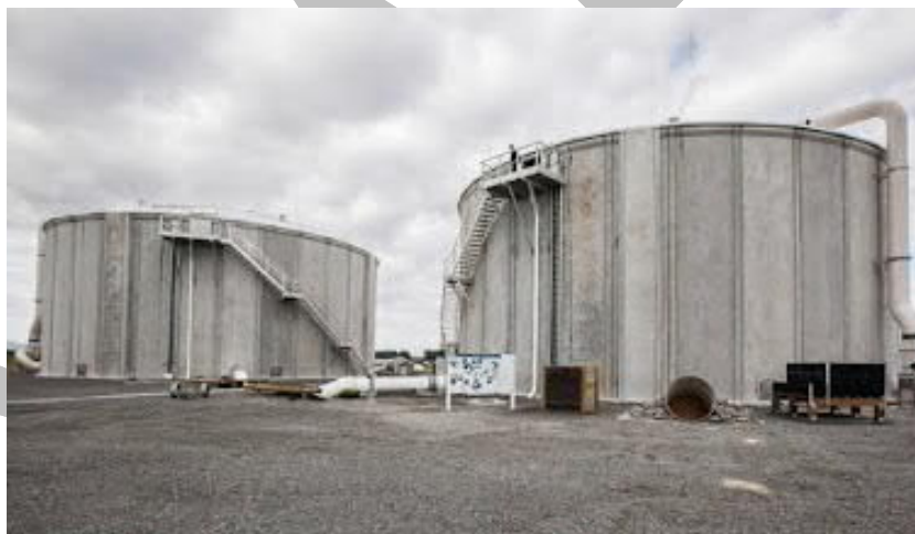
Photo 2 Napier Wastewater Treatment Plant Biological Treatment Filters
